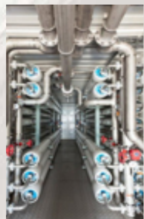
Reverse Osmosis System
